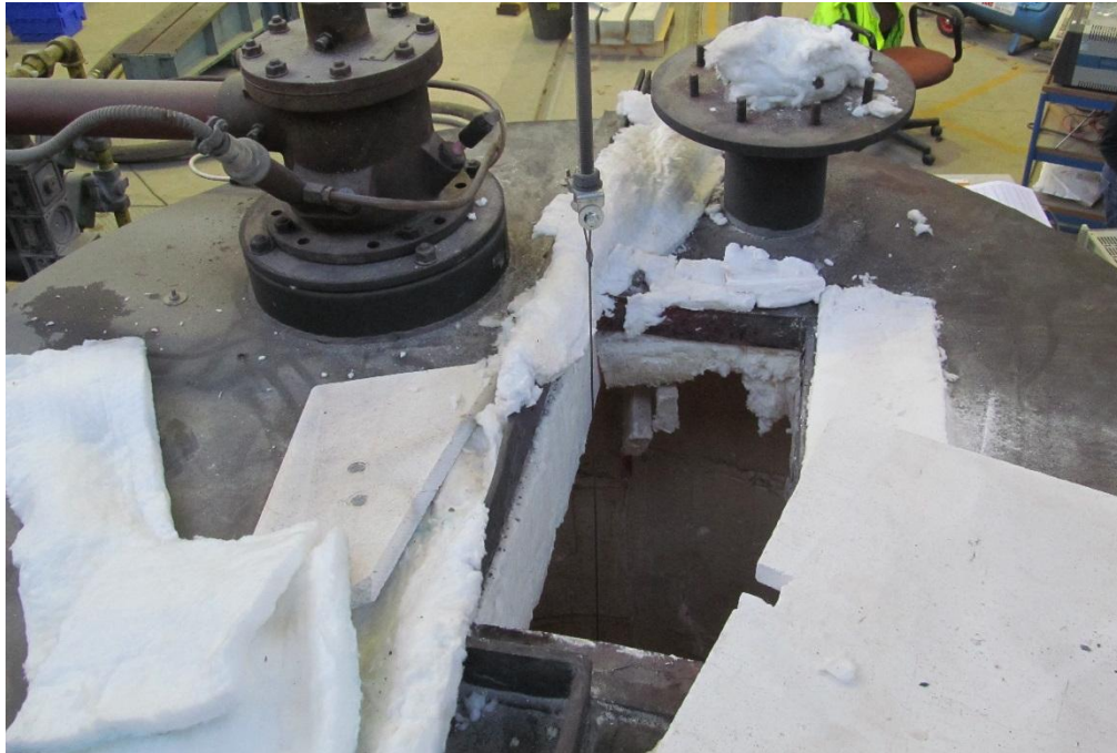
Figure 2 - Looped cable end suspended via threaded bar above the furnace
